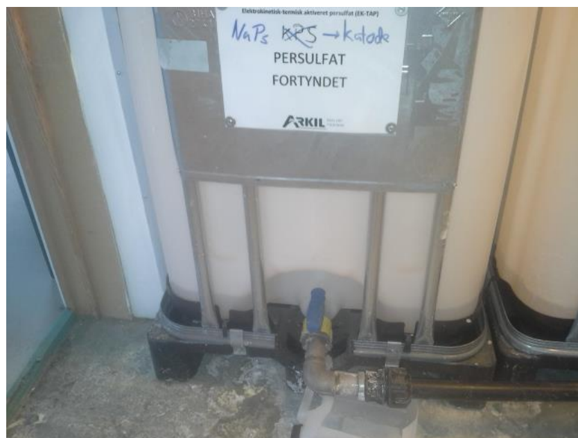
Figure 8.3: Connection of the buffer tank and the persulfate tank recycling content to CW.
