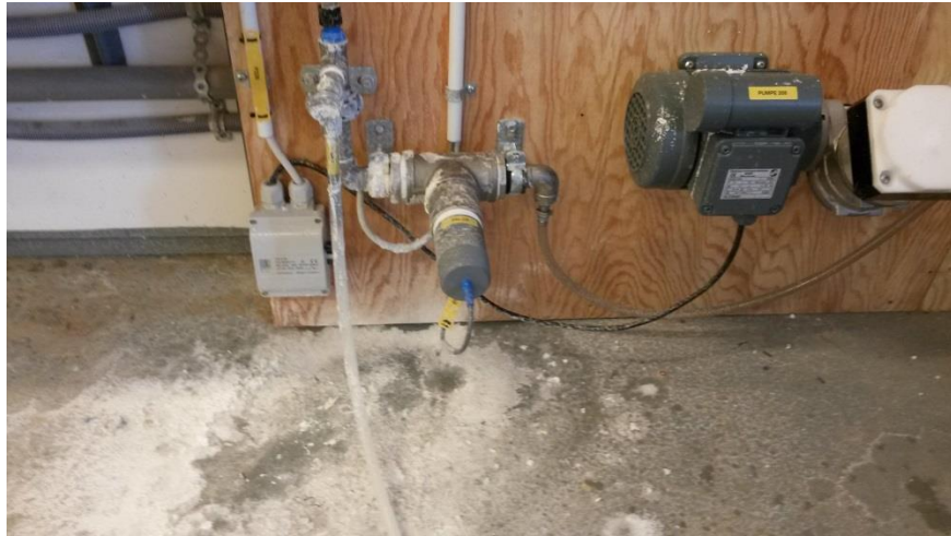
Figure 11.1: Operation leaks during the test period.
